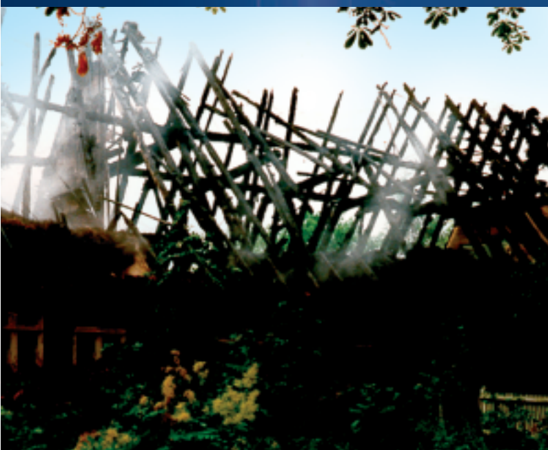
Lightning strike in the historical Worpswede town hall. Damage: approx. €1.7 million.
